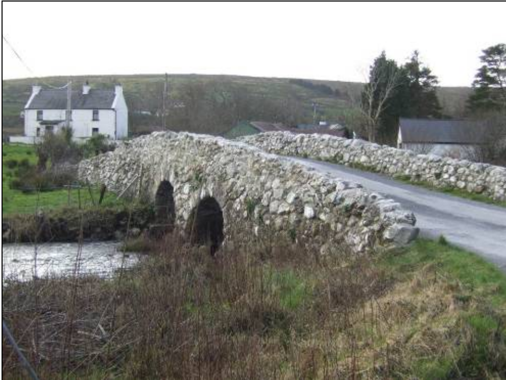
Image 13.6 BH 104 (with BH 103 in background), 'The Quiet Man' Bridge (Ch. 44+500 to Ch. 44+800), facing SSW
